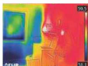
Uninsulated Outside Wall
