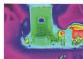
Infrared Thermograph for Power Circuit Board
